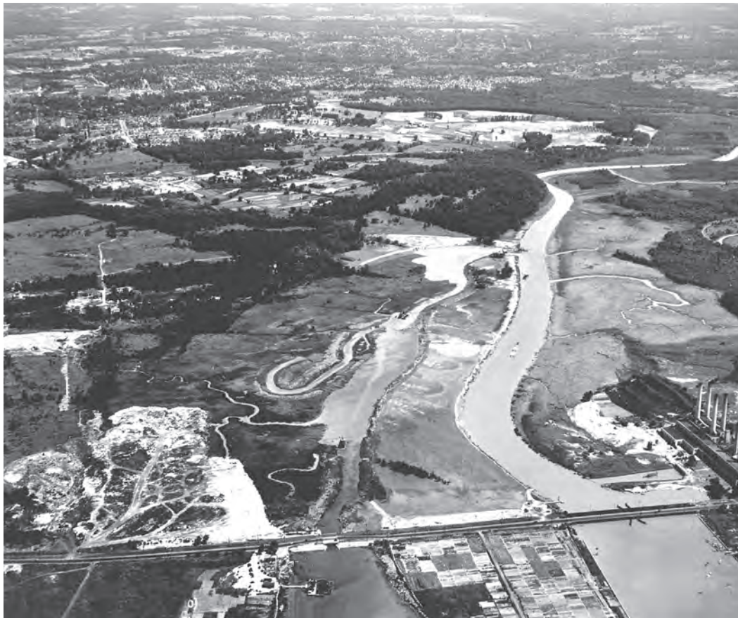
Anacostia Reclamation Project, July 1929. This aerial photograph shows the work on Section G of the project. Office of History, Corps of Engineers
