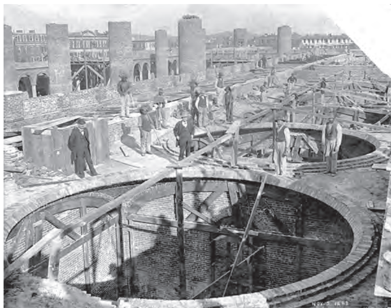
Pension Building under construction showing holes for shallow domes on the third floor, November 1883
