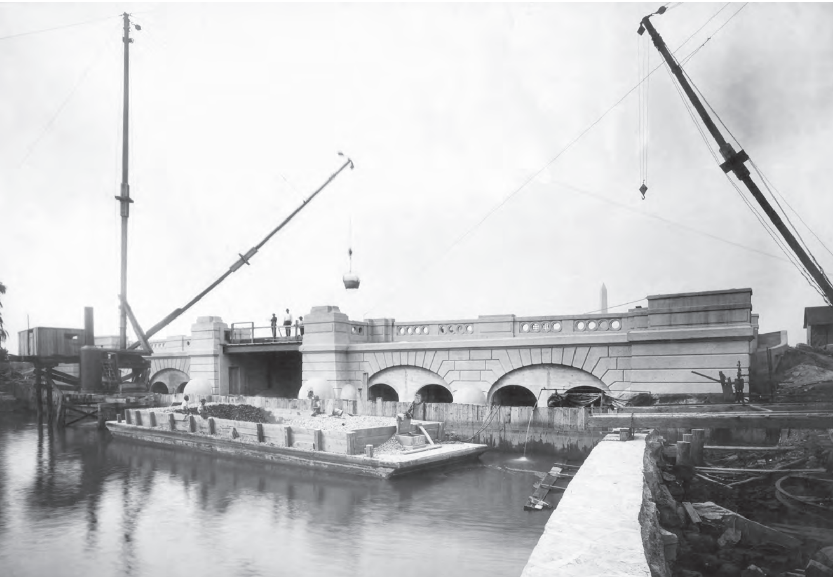
Construction of the inlet bridge for the Tidal Basin, 1909. The inlet and outlet bridges served as actual bridges at the same time their substructures were designed to flush out the Washington channel with each tide. National Archives no. 77-H-3334-45
