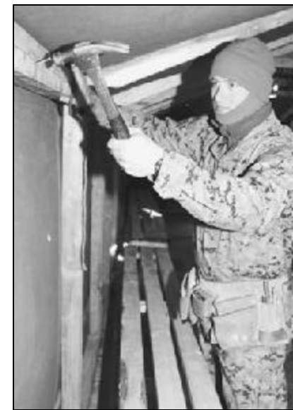
Lance Cpl. Nathan M. Thomas, MWSS-171 combat engineer, hammers in a nail to reinforce a strongback in the medical center in Korea for Exercise Foa Eagle 2005.
