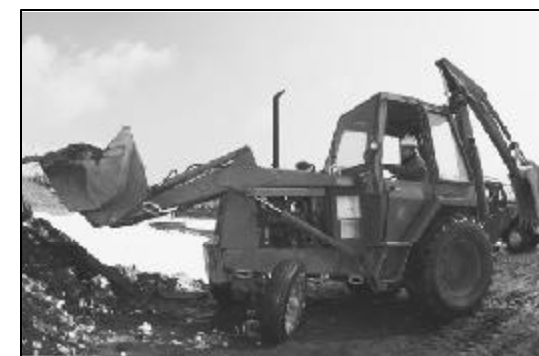
Pfc. Mark Fayloga Pfc. Joshua J. Henderson, Marine Wing Support Squadron 171 heavy equipment operator, helps out Camp Fuji's Navy Mobile Construction Battalion 40 with renovating outdoor basketball courts by excavating dirt where the new courts are to be placed, March 2.
