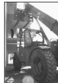
Lance Cpl. Lukas J. Blom A Military Millennium Vehicle-Skytrak hoists equipment to assist in barracks renovations.
