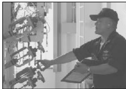
Petty Officer 2nd Class Astor Mojica, cryogenic technician, operates a generating plant that takes the impurities out of the processed air.
