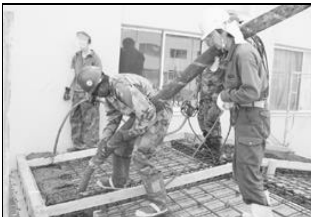
Petty Officer 3rd Class Ian Ferdinand, Naval Mobile Construction Battalion 5 laborer, places concrete for a canopy with a local contractor.
