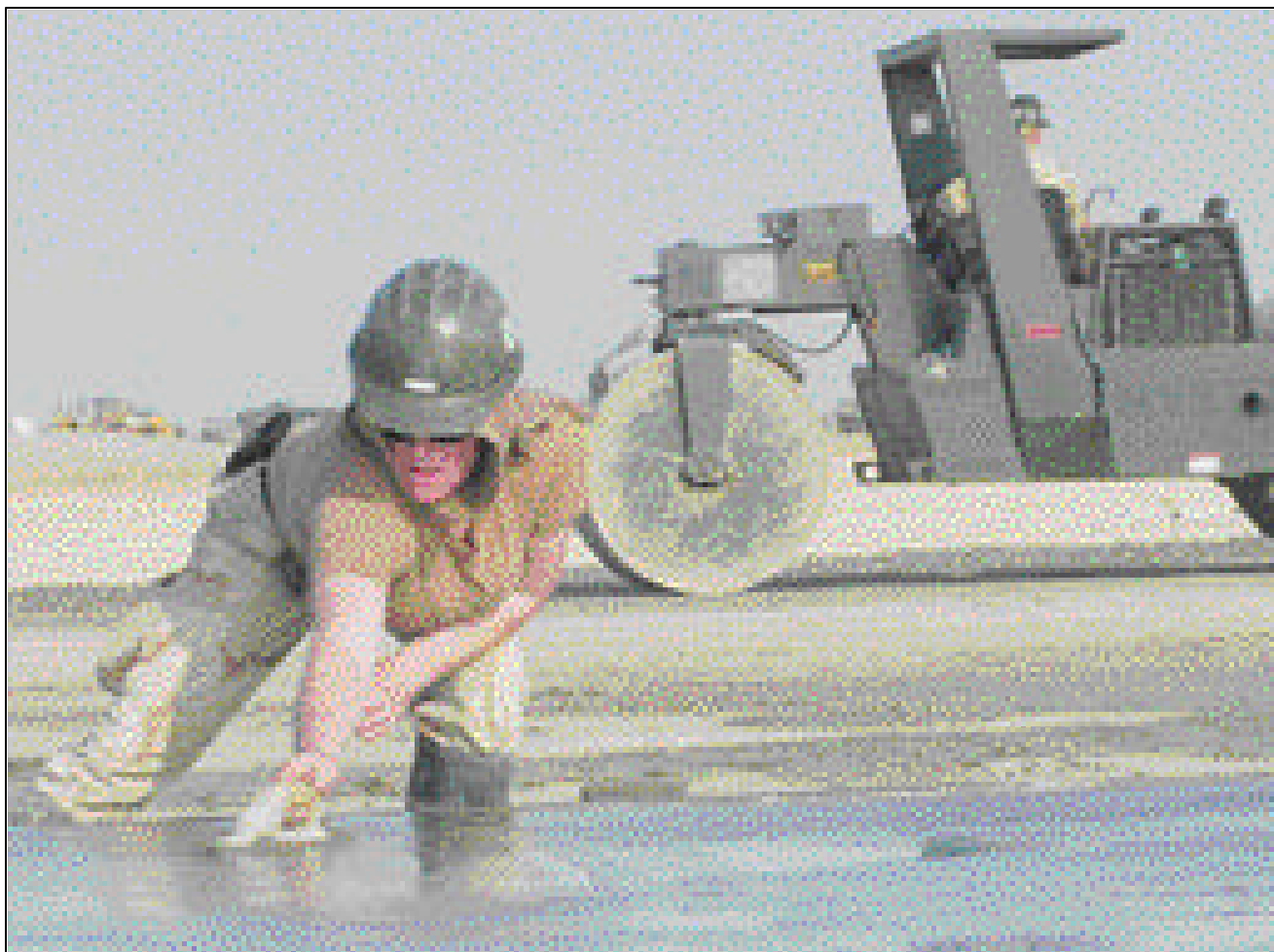
A Seabee deployed to Iraq smooths out a patch of concrete during their project to build a launching pad.
