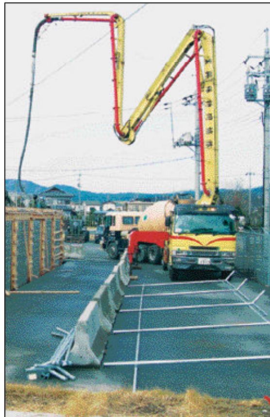
From small jobs to big jobs, Seabees are known for getting the job done. Their legacy was first established 1941 and continues to grow with every construction site complete and every mission met.
