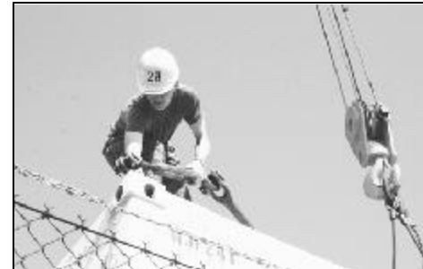
Lance Cpl. Justin Hager, MALS-12 mobile facilities technician, hooks a sling to the corner of the mobile facility in preparation for lifting.
