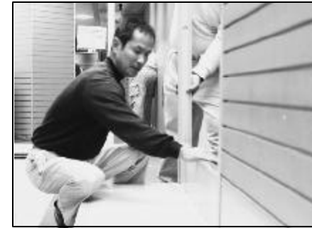
Norio Takase, employed with the maintenance department, builds a new shelf as part of the Seven-Day store expansion project.
