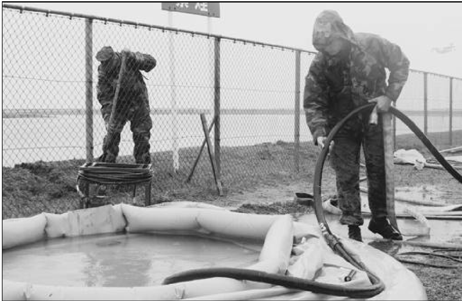
Pfc. Ryan Murphy drains water from a depleted holding tank. The holding tank is capable of retaining 3,000 gallons of water.
