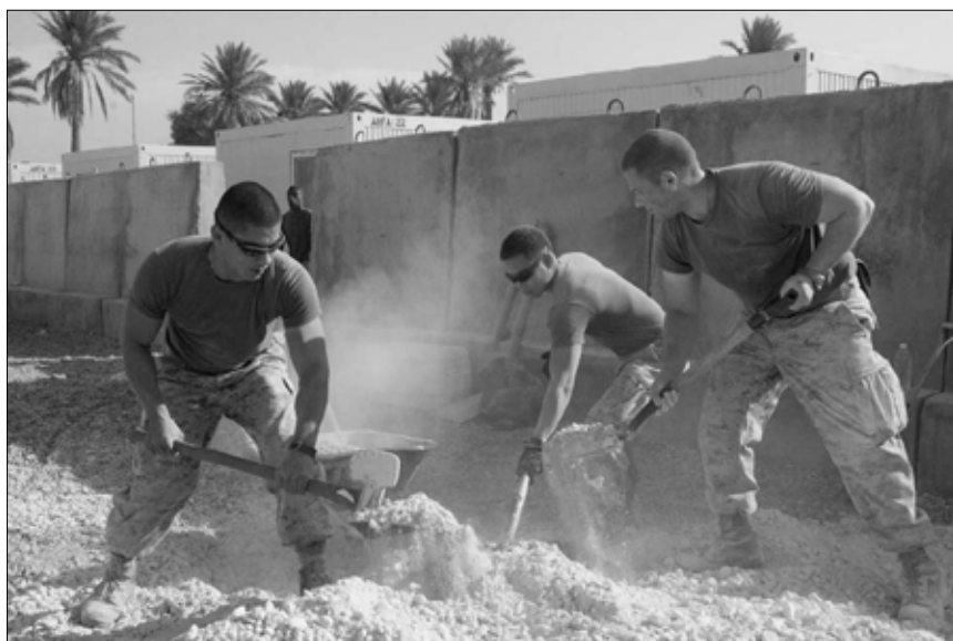
Marines with Regimental Combat Team 1 shovel gravel near their living quarters at Camp Ramadi, Iraq, Nov. 21. With only a couple of months left on their deployment, Marines are trying to put the finishing touches on the improvements to leave their facilities in good shape for incoming units. Photo by Army Sgt. Amanda Gauthier
