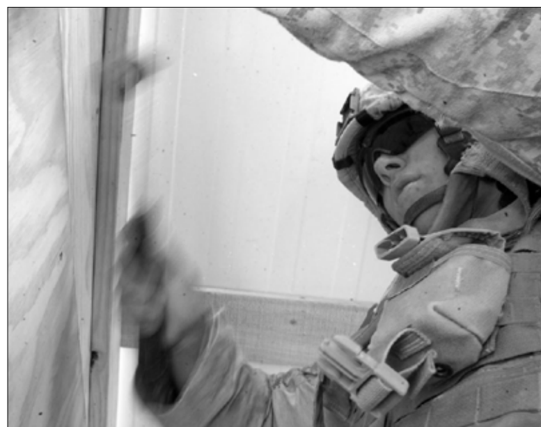
Lance Cpl. Kevin M. Kackos, 20, a generator mechanic with Support Platoon, Company B, 1st Combat Engineer Battalion, Regimental Combat Team 5, installs a wire fastener Nov. 18 in a newly constructed building built by the platoon near Rutbah, Iraq. Kackos is one of four utility Marines within the platoon who provides electrical and generator maintenance support for the platoon as well as for RCT-5. Photo by Cpl. Shawn Coolman
