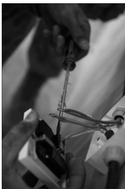
Lance Cpl. Dmitri R. Murray, 19, an electrician with Support Platoon, Company B, 1st Combat Engineer Battalion, Regimental Combat Team 5, fastens an electrical wire in a newly constructed building Nov. 18 near Rutbah, Iraq. Murray, along with three other utility Marines within the platoon, provides electrical and generator maintenance for the platoon as well as for RCT-5. Photo by Cpl. Shawn Coolman
