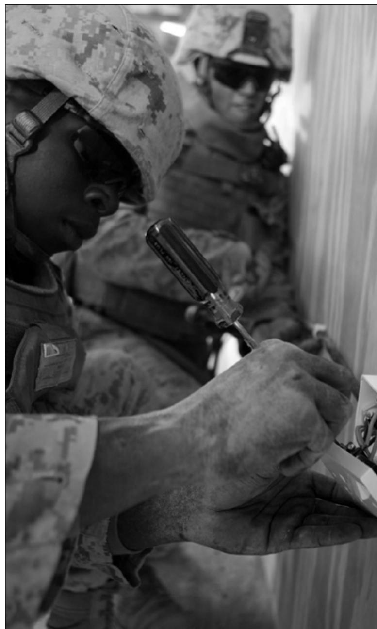
Lance Cpl. Dmitri R. Murray, 19, an electrician with Support Platoon, Company B, 1st Combat Engineer Battalion, Regimental Combat Team 5, connects the final wire on an electrical outlet while Lance Cpl. Kevin M. Kackos, 20, a generator mechanic with Support Platoon installs a wire fastener to hold the electrical wires in place Nov. 18 near Rutbah, Iraq. The two utility Marines are wiring a newly built building inside a recently built traffic-control point built by the platoon. Photo by Cpl. Shawn Coolman
