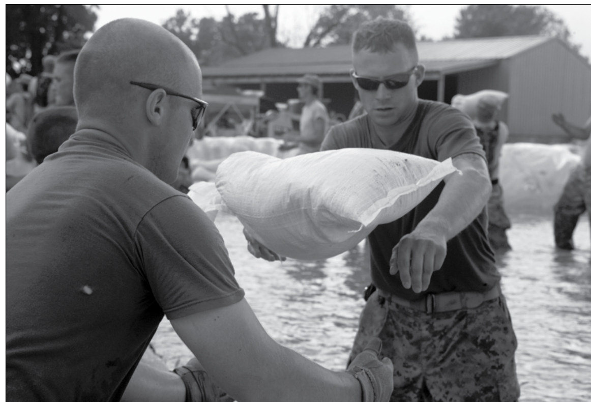
Marines and sailors of 26th Marine Expeditionary Unit stack sand bags to reinforce the levees June 9 in Elnora, Ind. Local authorities in Elnora requested the 26th MEU to provide support to reinforce the levees from flooding of the White River. Photos by Cpl. Jason D. Mills
