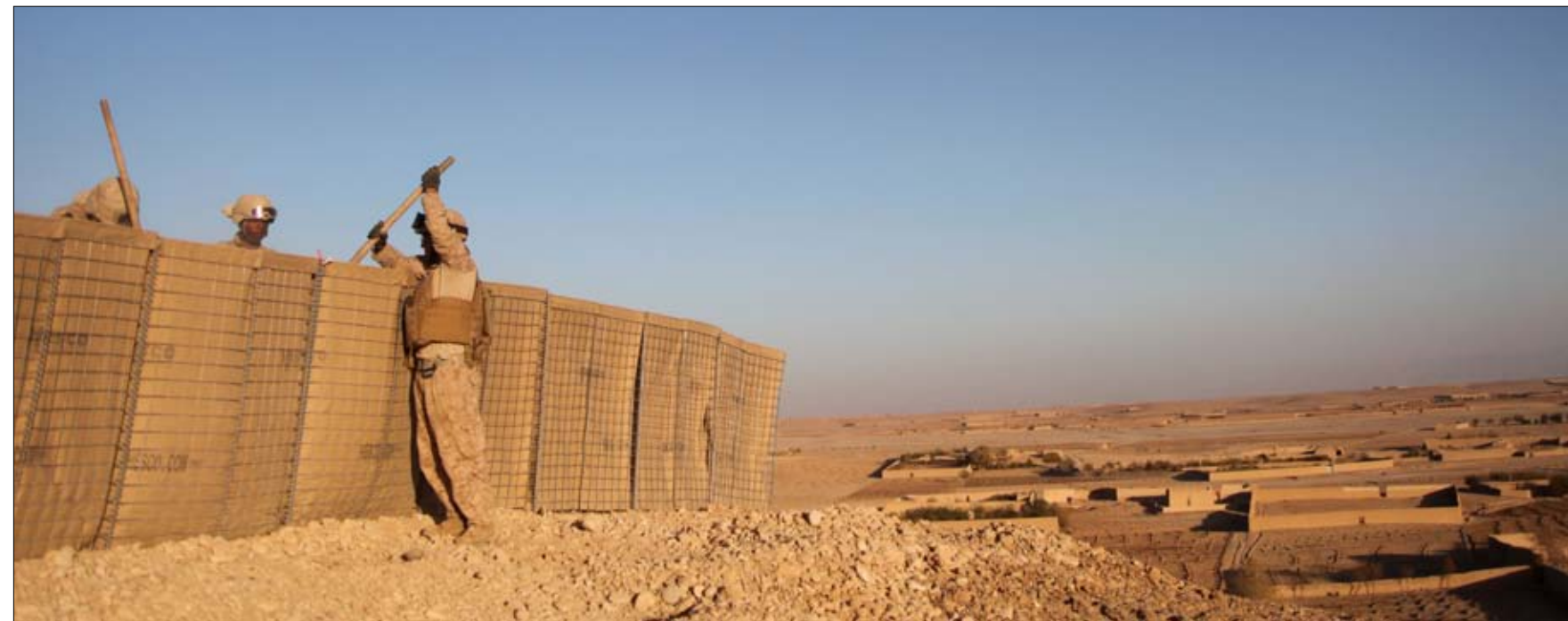
MUSA QAL'EH, Afghanistan — Engineers with 1st Combat Engineer Battalion, 1st Marine Division (Forward), fill Hesco barriers at a new combat outpost in Musa Qal'eh, Nov. 13. Afghan forces were in need of a defensive position due to enemy activity in a nearby town.
