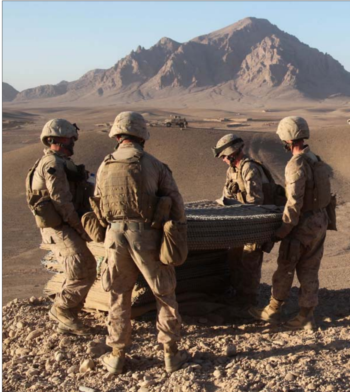
MUSA QAL'EH, Afghanistan — Engineers with 1st Combat Engineer Battalion, 1st Marine Division (Forward), move a stack of Hesco barriers at a new combat outpost in Musa Qal'eh, Nov. 13. Building an elevated position at the top of a hill allows Afghan forces the ability to watch over the surrounding area.
