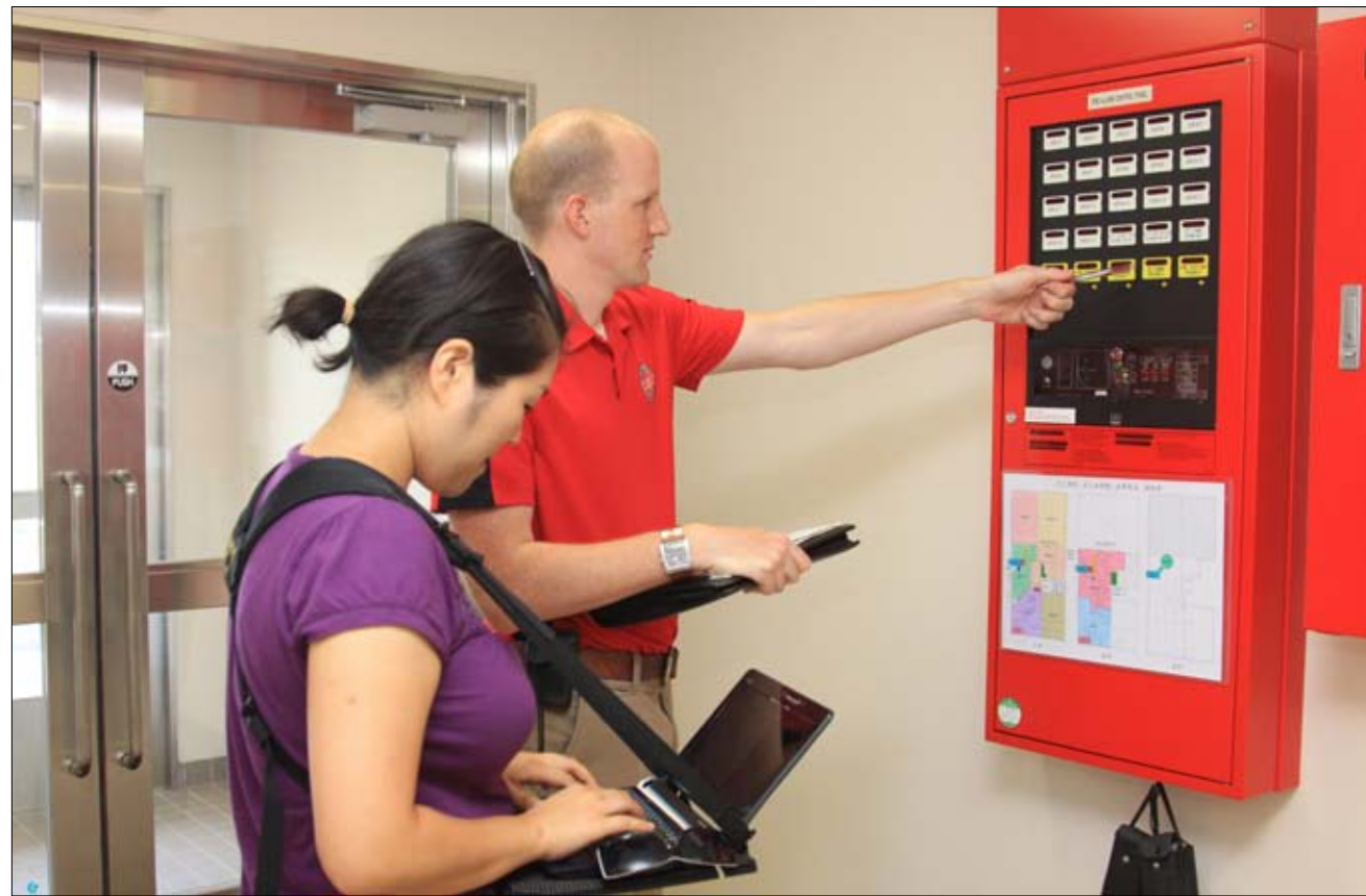
Brendan Donnelly and Mi Sun Kim, fire protection engineers, evaluate a fire alarm panel in the Aircraft Rescue Firefighting facility here Sept. 2. Donnelly explained the structure of the panel while Kim gathered the information on a computer attached to an engineer's "connect a desk" device.
