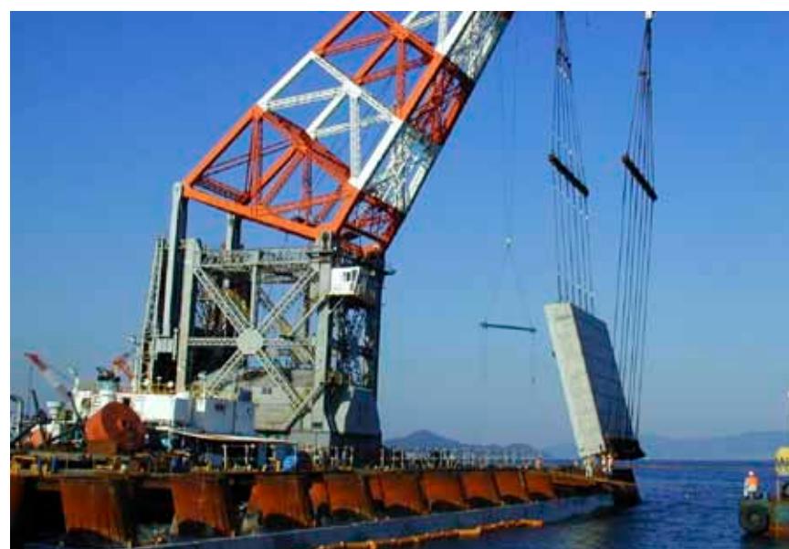
PHOTO COURTESY OF THE CHUGOKU-SHIKOKU DEFENSE BUREAU A large cement block is lowered by a large crane as a base for the south side seawall during the construction of the newly finished runway. Construction of the runway was accomplished in three phases. Phase one involved the construction of a new port facility which was completed in 2005. Phase two involved the construction of the north end of the runway while phase three concentrated on the middle.
