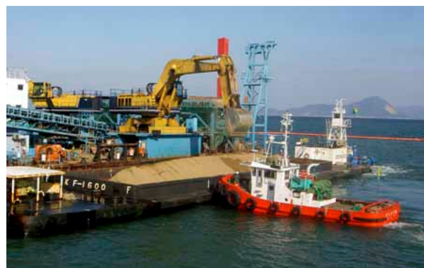
PHOTO COURTESY OF THE CHUGOKU-SHIKOKU DEFENSE BUREAU A crane transports soil from a barge onto a conveyor belt during the process of building the newly finished runway. Construction of the new runway involved the joint efforts of the government of Japan, the Ministry of Defense, the Chugoku-Shikoku Defense Bureau, the Japanese construction industry, the U.S. Army Corps of engineers, the Naval Facilities Engineering Command Pacific, the Marine Corps Air Station Iwakuni Facilities Department and others.
