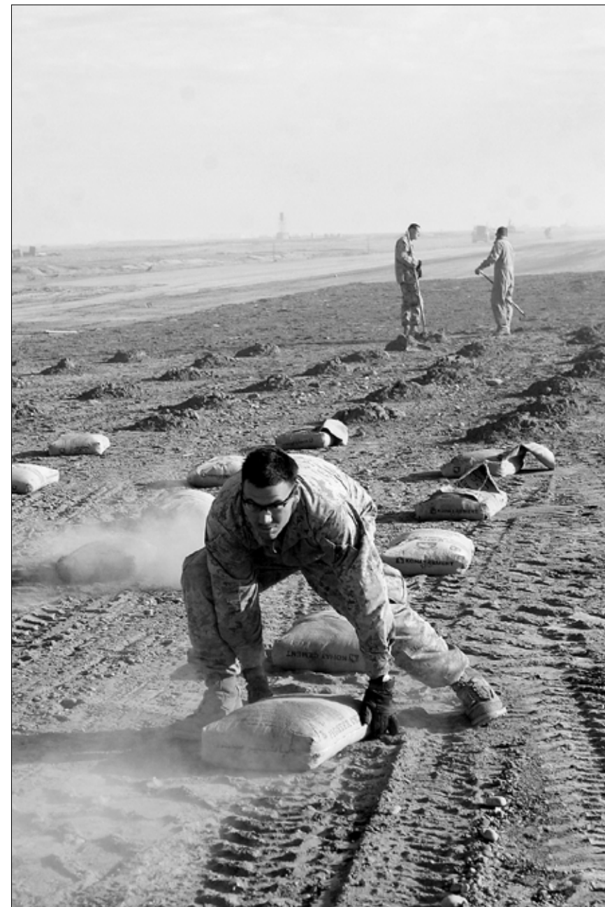
CAMP DWYER, Afghanistan — Lance Cpl. Travis Vliet, a combat engineer with Marine Wing Support Squadron 372, Marine Aircraft Group 40, Marine Expeditionary Brigade-Afghanistan, covers and aligns a bag of concrete for the expansion of the C-130 runway here, Jan. 23.
