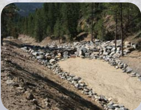
A sediment trap, which reduces metals and sediment flowing from orphan mine sites, is ready for clean out.
