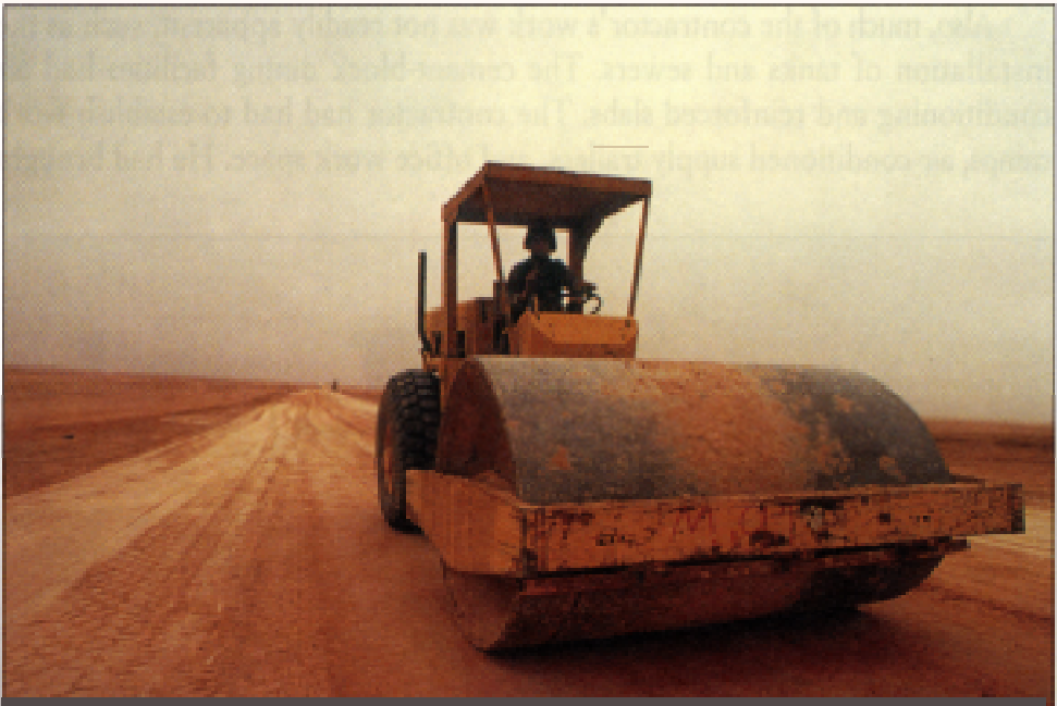
Soldiers from the 20th Engineer Brigade compact the ground for a new road in Southwest Asia.
