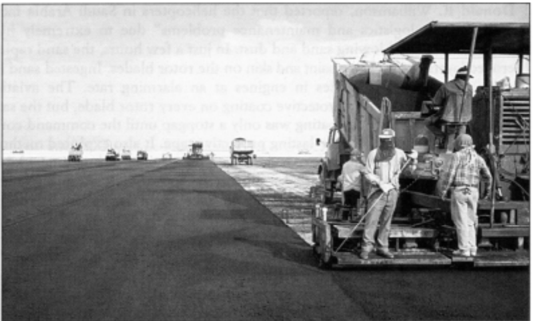
Two asphalt paving machines work side by side at the King Fahd International Airport. Five of these machines were used simultaneously to handle the daily requirement of
