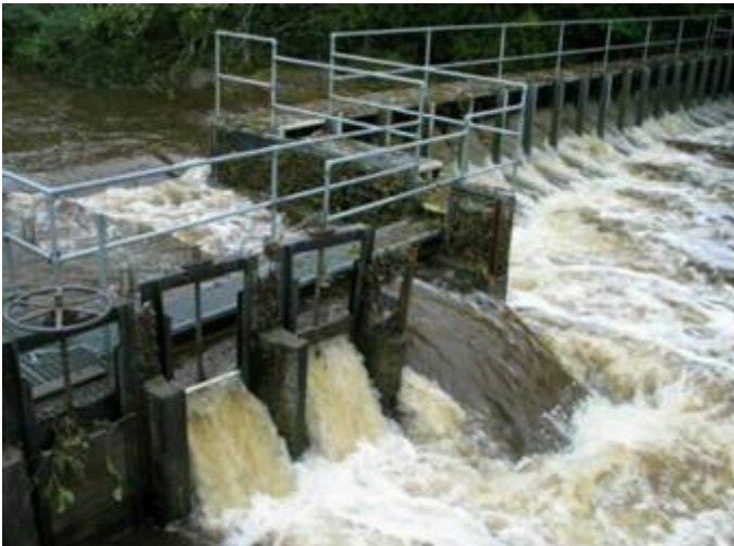
Figure 11 -- Failure of weir to restrict passage during a period of high flows on Minter Creek, WA.
