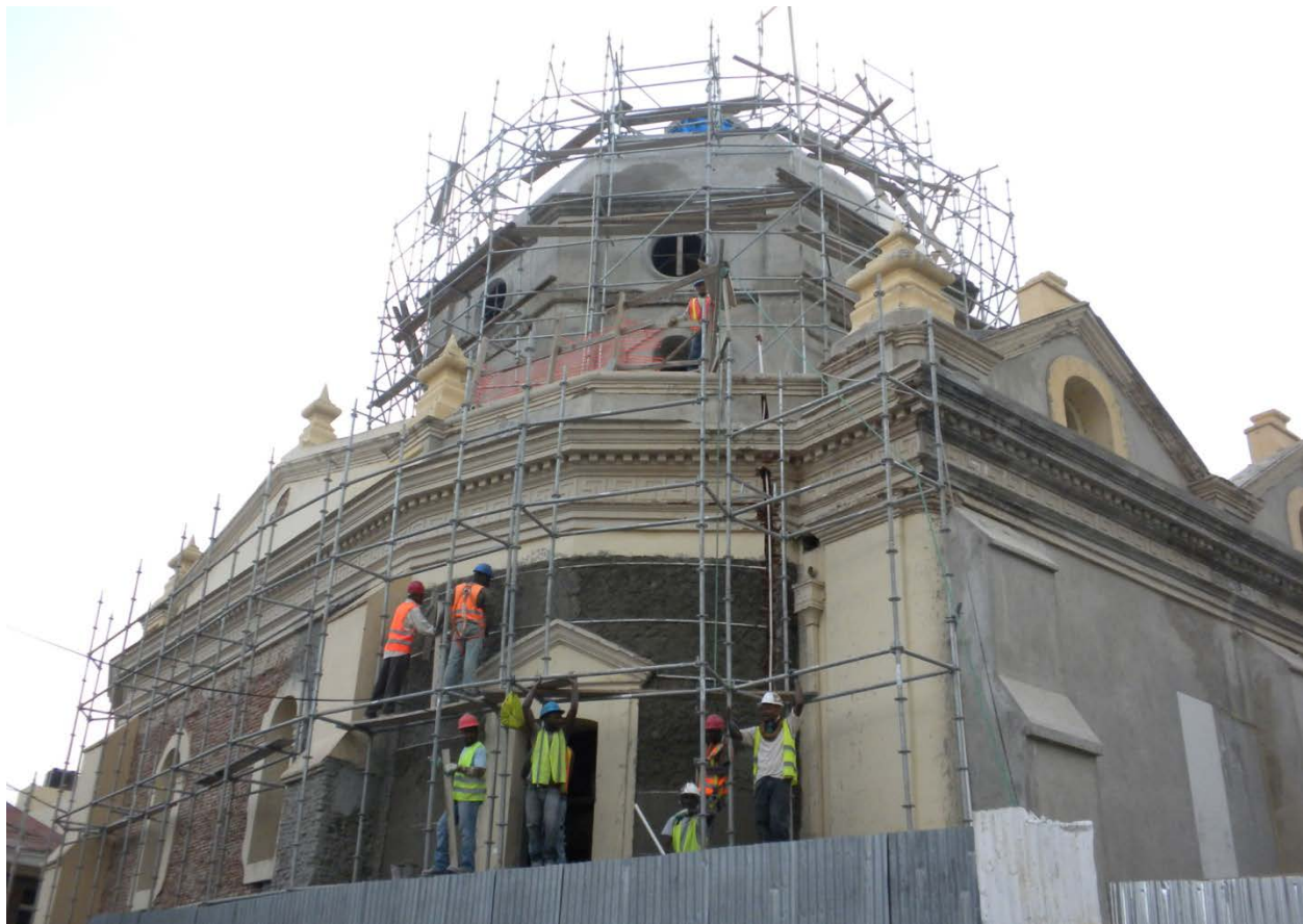
Image 2: Haitian and Dominican construction workers with the government contractor Acero Estrella are busy working on the renovation of the cathedral in Santiago de los Caballeros.
