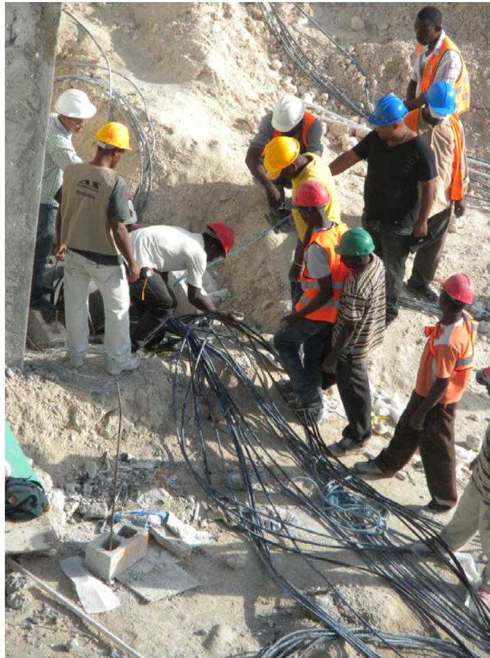
Image 3: As Haitian construction workers become more qualified, they are present in greater numbers in the technical phase of the construction project, as seen here in the installation of wiring in a hotel in Punta Cana.
