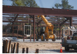
Heavy equipment moves steel beams into place Feb. 14, as construction on the new Warrior Transition Unit gets underway at Fort Gordon.
