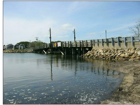
This wooden drawbridge in Chatham is one of a very few such structures still in existence in the nation and is unique in Massachusetts. (Photo courtesy Friends of the Mitchell River Wooden Drawbridge)
