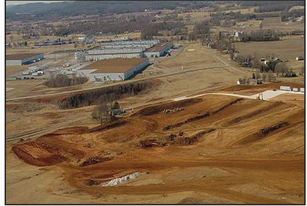
Aerial photo of construction in Phase I of the Kentucky Transpark industrial development (840 acres). The Phase I development is just west of the proposed connector road. Phase II (340 acres) will be built to the east of the road.
