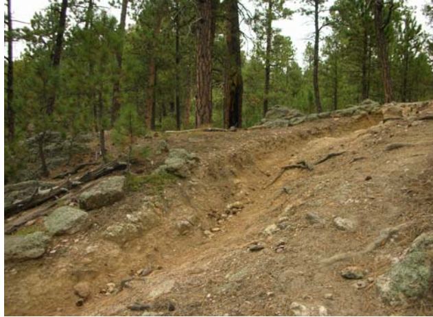
Figure 31. Horse trail erosion (photo by National Park Service).
