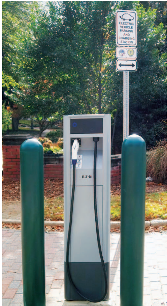
Raleigh, North Carolina, is among the many U.S. cities installing EVSE in public places. Photo from Kathy Boyer, Triangle Clean Cities Coalition, NREL/PIX 18520
