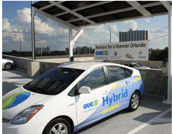
Public charging stations that incorporate renewable energy, such as these solar panels, can be particularly appealing to environmentally conscious drivers. Photo from IKEA Orlando, NREL/PIX 18709
