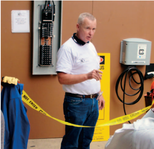
The Electric Vehicle Infrastructure Training Program is one of the organizations that trains electrical contractors in EVSE installation. Photo from Electric Vehicle Infrastructure Training Program
