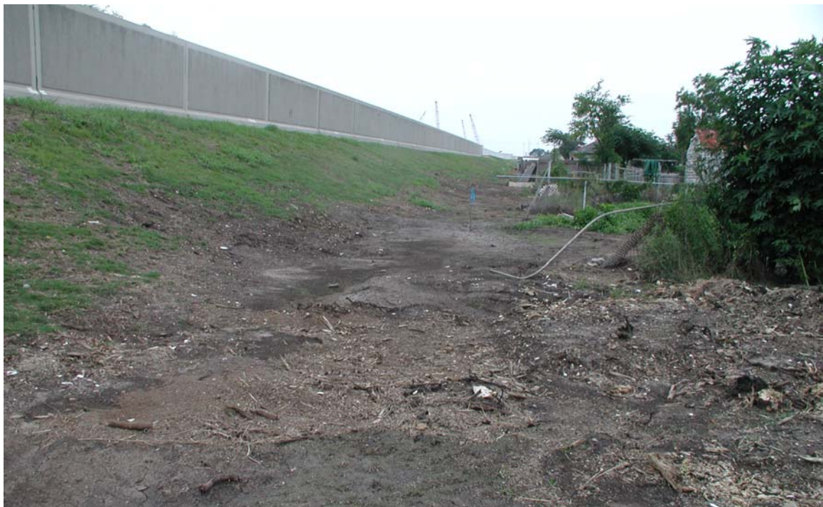
Figure B-15 – View of Protected Side Toe of Levee in Test Area Looking North
