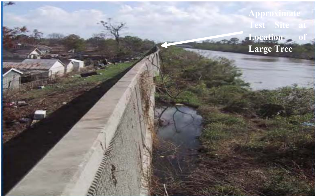
Figure 31. Tilted I-Wall Opposite the North Breach on the London Avenue Canal
