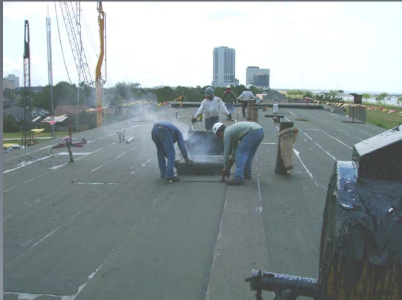
Workers install a new roof at the Bonnabel Pump Station in Jefferson Parish.
