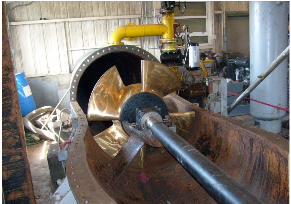
This horizontal pump was included in the repairs to the Hayes Pump Station in Plaquemines Parish. Other repairs at Hayes included two new diesel drive engines and two chain drive pumps.
