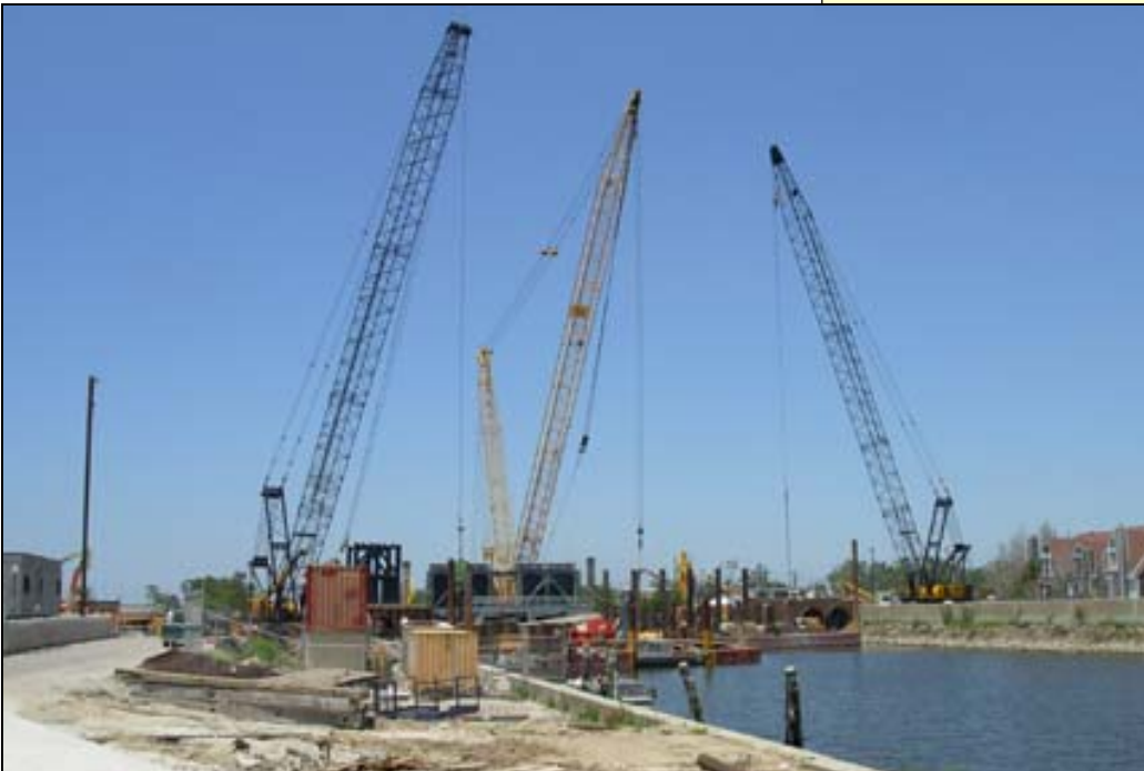
Installation of the pumps and gates at the 17th Street Canal continues. Photograph by Todd Hornback.
