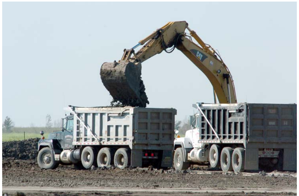
Trucks get loaded with borrow material (levee dirt) that will be driven to a levee construction site. Approximately two million truck loads of borrow will be moved over the next two years to complete the HSDRRS. (USACE Photo)
