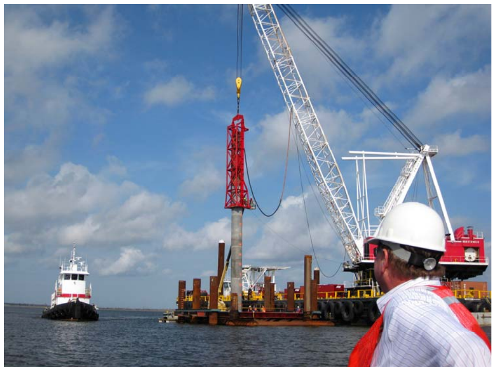
Shaw Environmental & Infrastructure crews drive piles for the IHNC Lake Borgne Surge Barrier. (Photo courtesy of Shaw)
