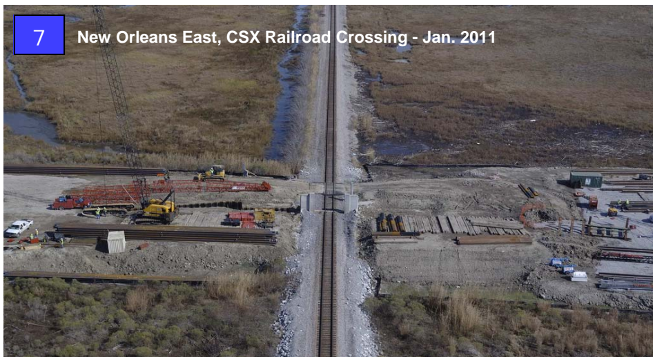
Crews work to replace the existing railroad gate where it intersects with the levee just north of the GIWW.
