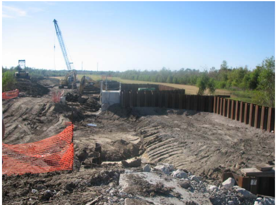
Work has started on the Almedia drainage structure in St. Charles Parish. This section of levee is being retrofitted to raise the levee to 15.5 feet, the 100-year level elevation.
