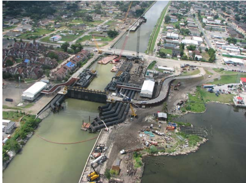
17th Street temporary pump station
