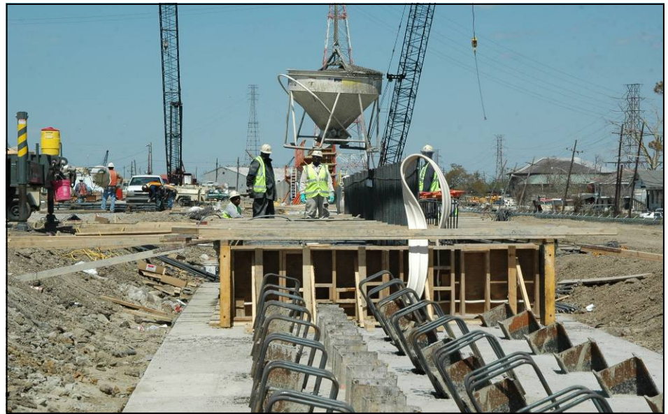
Rebar, H-beams and concrete were the main construction materials used for repairs and improvements of the Inner Harbor Navigation Canal floodgate. (USACE Photo)
