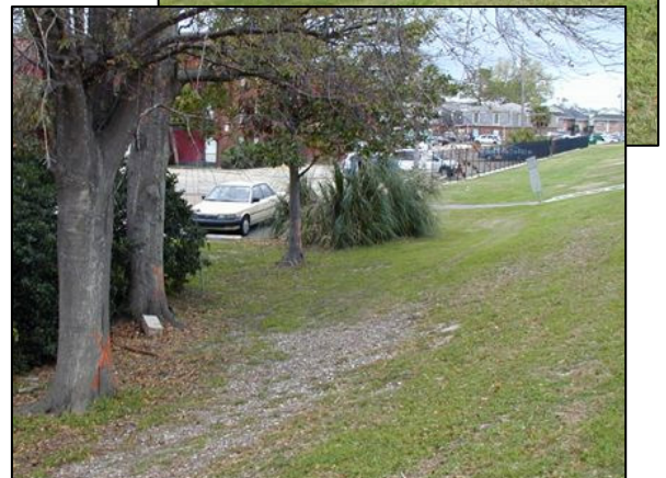
The top photograph shows a tree that has grown in the levee. Above, these trees have grown at the levee toe.
