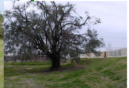
This tree stands within the levee toe.
