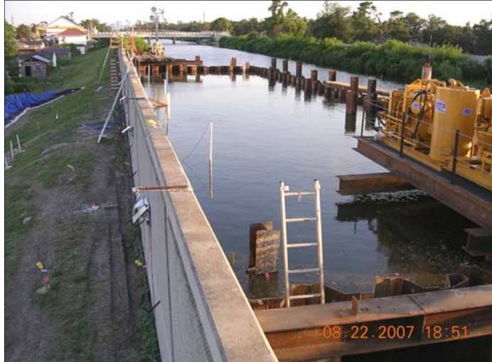
This photo of the cofferdam at London Ave. Outfall Canal was taken on August 22, the day the water level reached seven feet. (USACE Photo)
