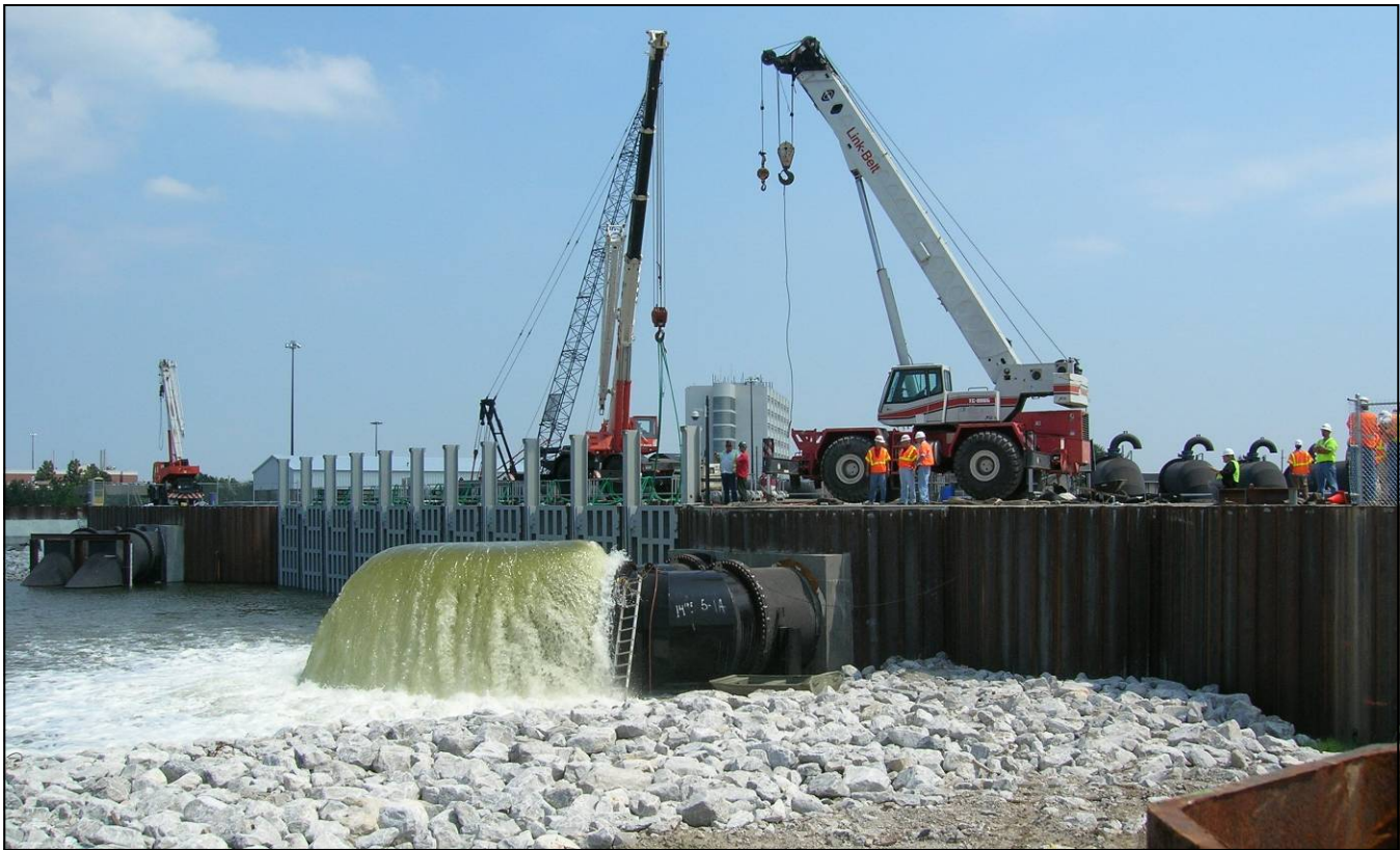
The Corps of Engineers conducts regular tests of outfall canal pumps as they are installed and as pumping capacity increases. This test was performed on Sept. 20 at the London Ave. Canal. (USACE Photo by Barry Fletcher)
