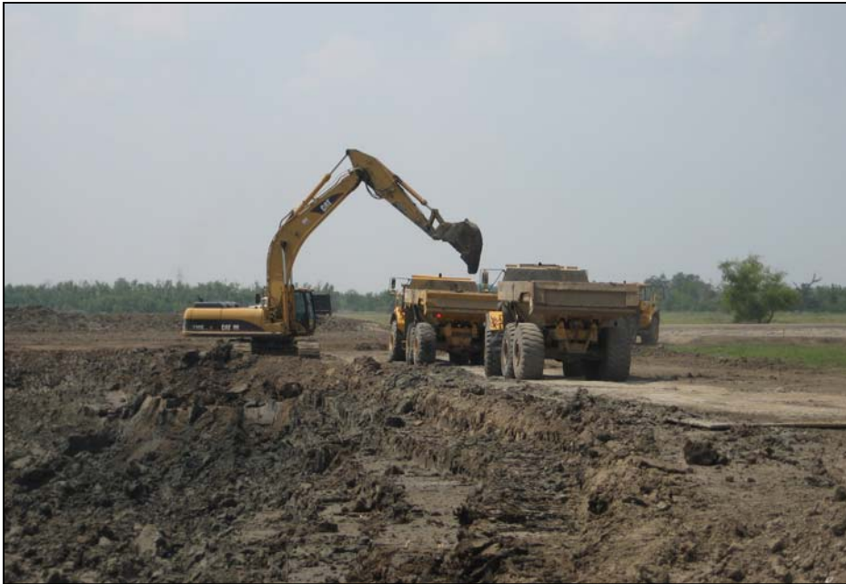
Crews gather clay for levee construction at the Myrtle Grove Borrow Pit in Plaquemines Parish. (USACE Photo by Paul Floro)
