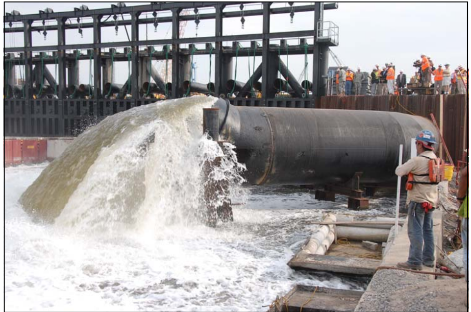
This photo shows one of the temporary pumps performing at a public demonstration last summer at the 17th Street Canal. (USACE Photo)
