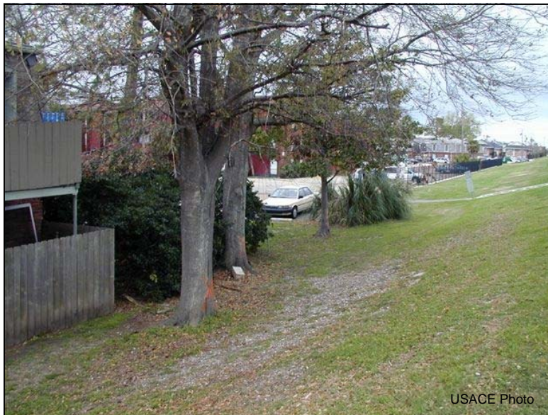
Trees and fences too close to the floodwall or levee toe must be removed to protect the integrity of the structure.
