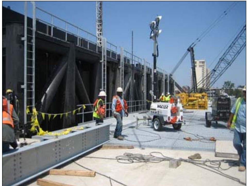
Construction continues at the 17th Street outfall canal where temporary pumps and flood gates are being installed. (USACE photo)
