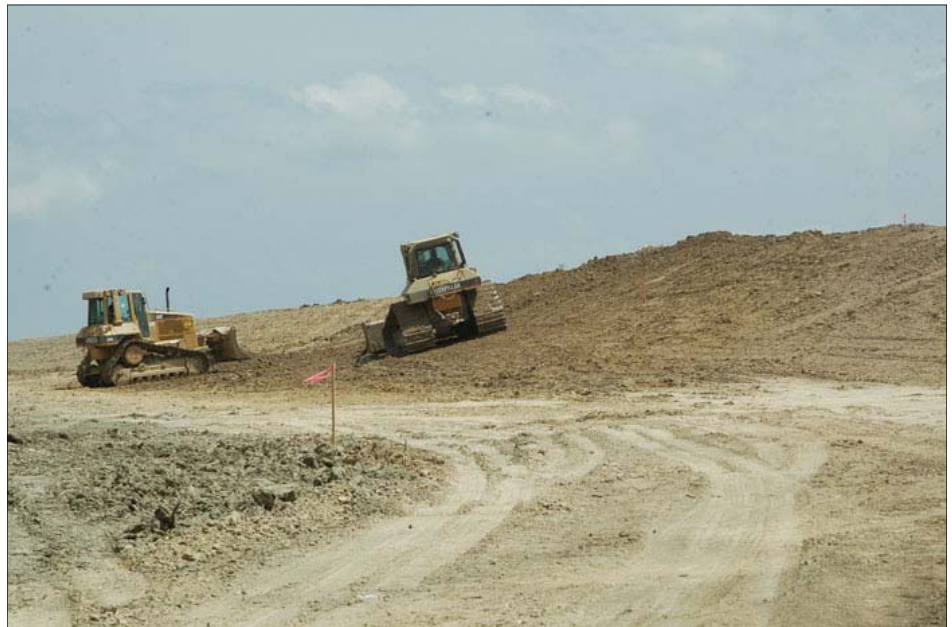
Bulldozers push soil material up an earthen levee to build a new levee lift. The material used for levees is clay soil that requires numerous tests before it is accepted for levee embankments. (USACE Photos)
