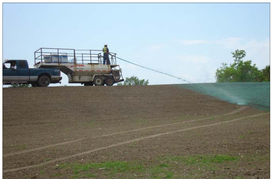
This levee is receiving hydro-mulching - spraying of grass seed, fertilizer and mulch all in one process.
