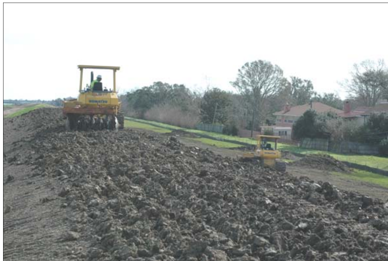
Bulldozers scarify a levee surface to prepare it for a new lift of clay. This process roughens the levee and allows the existing surface to bond and blend with the new lift. (USACE Photos)
