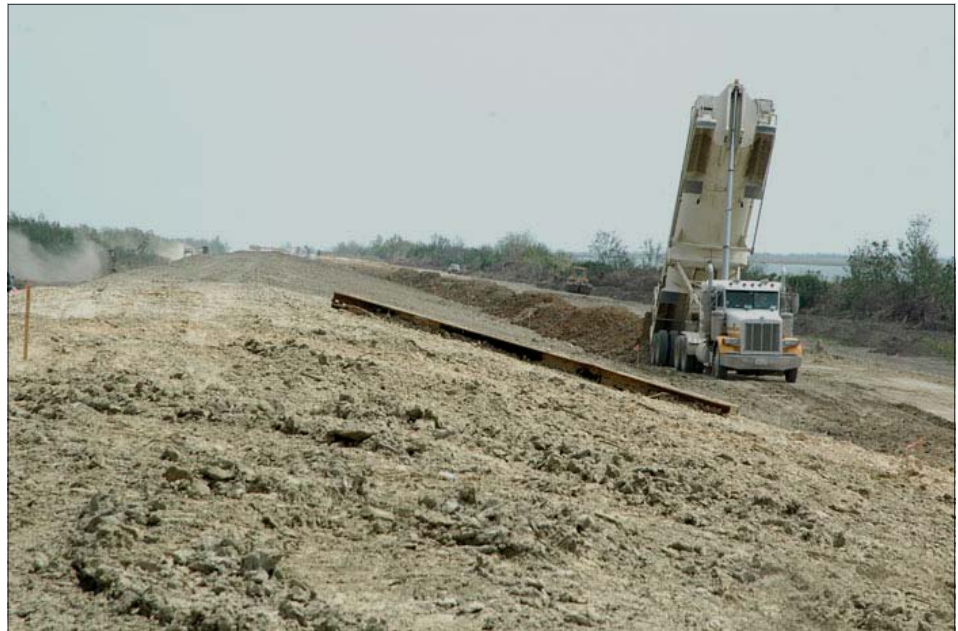
A dump truck empties its load of approved clay at a levee-building site.
