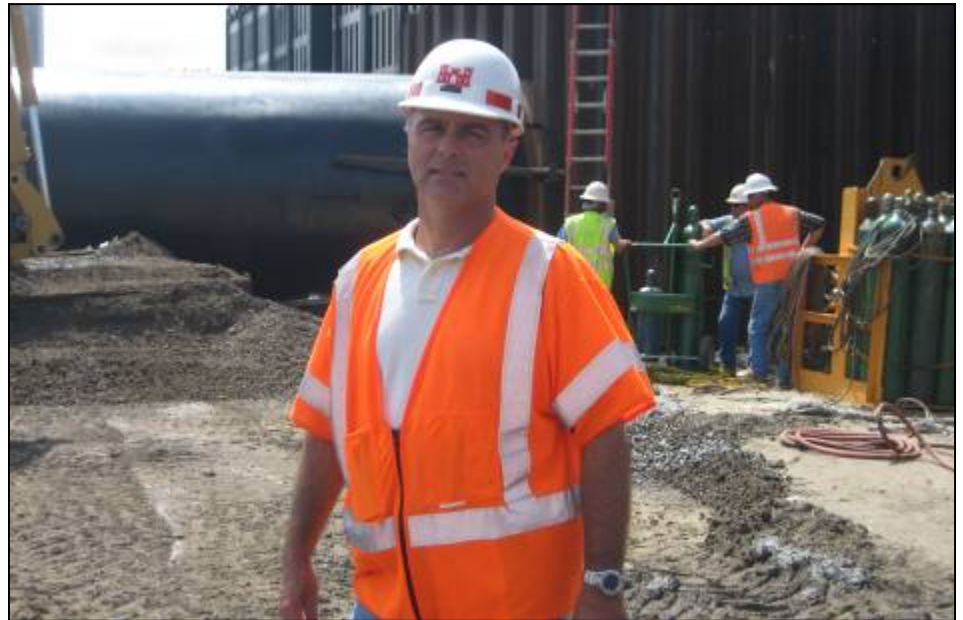
Maurice “Duke” Ducarpe represents the Corps of Engineers at the 17th Street Canal. Workers in the background are busy welding newly arrived pumps. Boh Brothers is the contractor on site.
