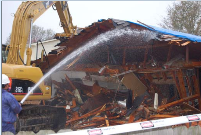
A LaRFO employee sprays water on a house demolition to reduce the risk of asbestos dust. (USACE Photo by Patty Mixon)
