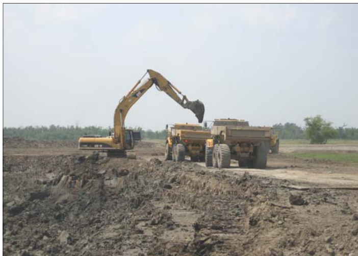
A backhoe places borrow (levee material) from a local pit into a truck for transport to a levee. The Corps will need 100+ million cubic yards of borrow to build the levees to the 100-year level of protection. (USACE Photo)
