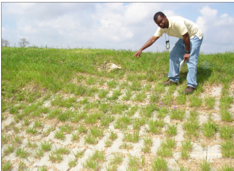
The Corps is experimenting with different types of matting materials to be used as armoring for levees. The material should be porous enough to allow grass to grow through it, like the articulated concrete blocks in the levee above. (USACE Photo)
