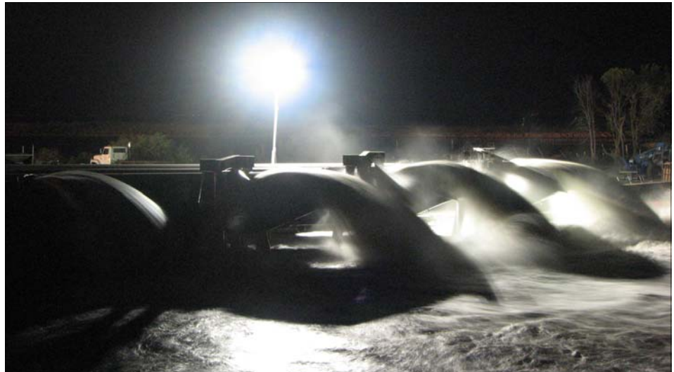
August 20, 2007 9:00 p.m. 17th Street Outfall Canal New direct drive pumps pushing 4,000 cfs of water into Lake Pontchartrain (USACE Photo by Paul Floro)
