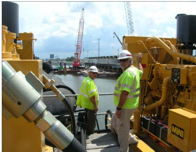
Inspecting installation of new pumps at the 17th Street Outfall Canal are Russ Wiggs, left, and Dennis McMurdo. (USACE Photos by Barry Fletcher)
