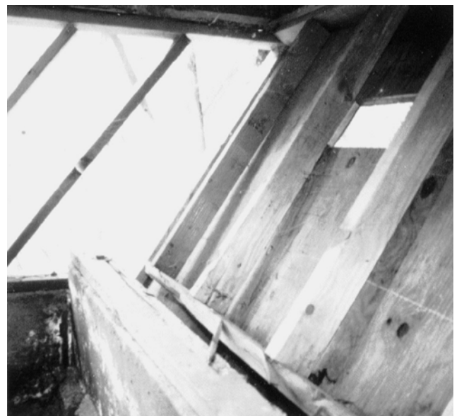
Figure 23 - This photograph shows an interior detail of a home similar to the one above, showing substantial damage to a building with an unbraced tall wall.
