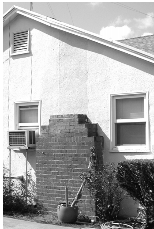
Figure 35 - Photo showing damaged chimney removed. Note that the fireplace is now not functional.
