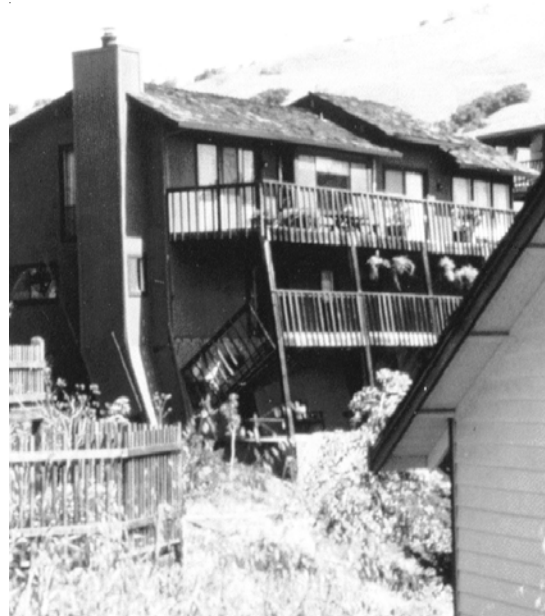
Figure 22 - This hillside home was built on an unbraced tall wall that failed.
