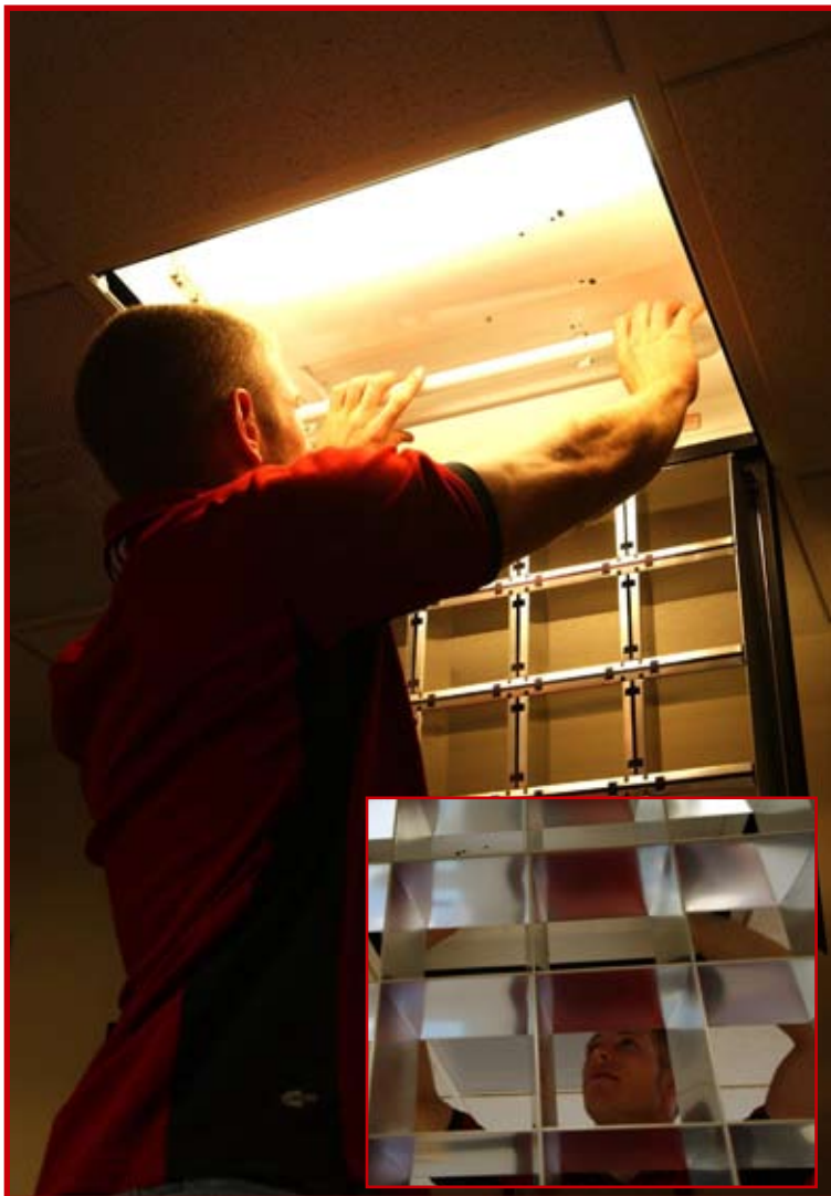
Dan Kontz replaces lightbulbs in the 931st Air Refueling Group Headquarters building. Kontz performs building and grounds maintenance for the 931st ARG. Kontz has been with the 931st ARG since Sept. 2004 and has been a civilian employee on McConnell Air Force Base, Kan., since the summer of 2003. Dan's father, Lt. Col. Keith Kontz, is the 931st ARG Chief of Standardization and Evaluation. (Air Force Photo/Staff Sgt. K.L. Kimbrell)
