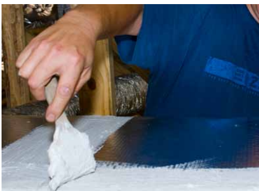
Mastic is a thick sealant that is painted on to rigid ducts to seal seams and joints (Source: FSEC).
