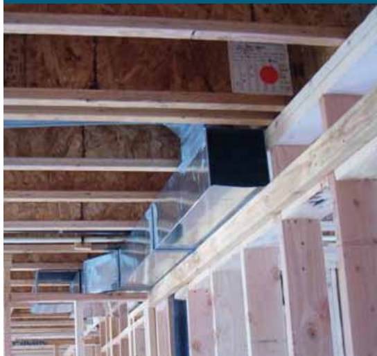
This Building America builder puts ducts inside the home instead of above the insulation where they would be exposed to cold and hot attic conditions.
