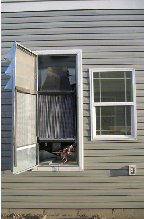
This evaporative cooler mounts on an exterior wall of a home built by Community Development Corporation of Utah with design assistance from Building America's Consortium for Advanced Residential Buildings (CARB) research team (Source: Steven Winter Associates).
